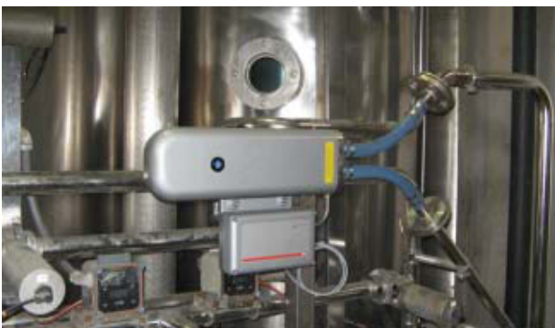
Fig. 7: DPRn 4122 density transducer at regeneration of de-acidification column
