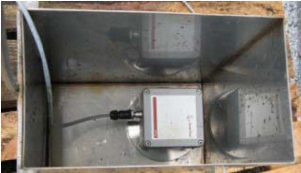
Fig. 3: SPRn 4115 L 2T mounted inside stainless steel box
